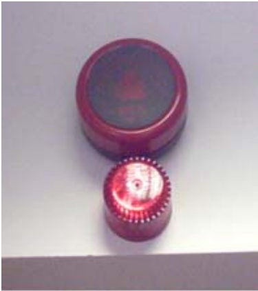
Figure 9 Dual Visual and Auditory Alarm System
